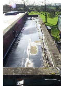
Burton upon Stather Primary School - Water ponding
